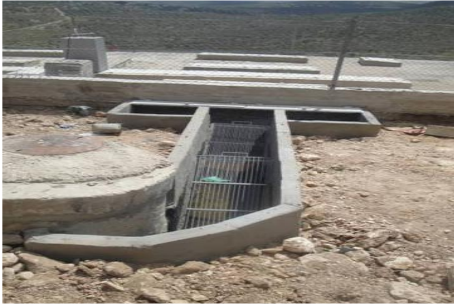
Photo 1. Headworks and UASB reactor of Bani-Zeid pilot
