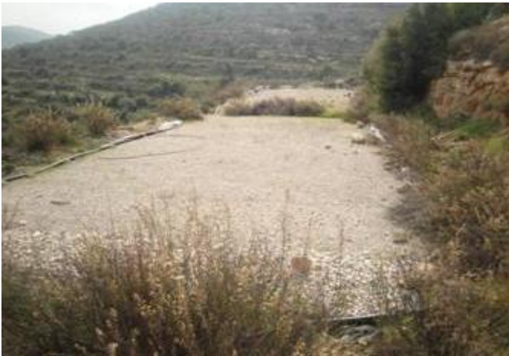
Photo 5. Constructed wetland basin of Bani-Zeid pilot WWTP
